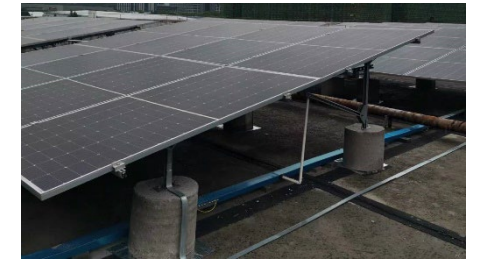
Nanjing Nikon Solar panels
